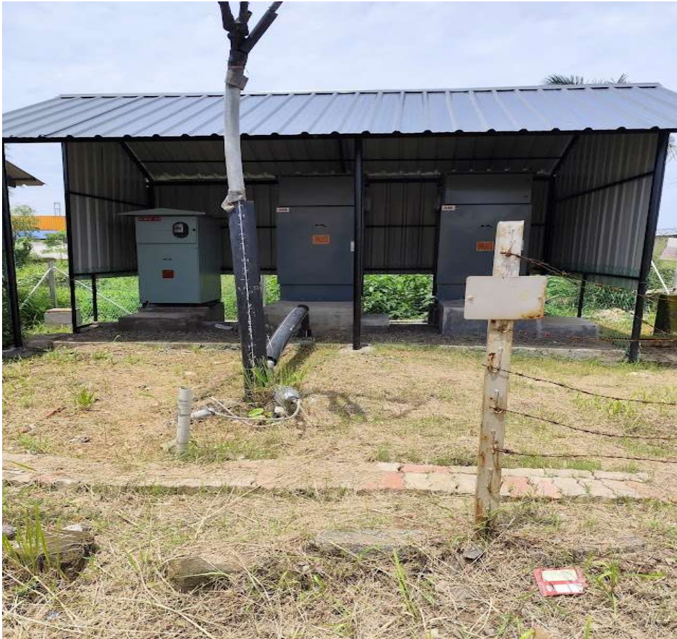
Incoming feeders from KSEBL at Vallarppadam 11 kV S/S
